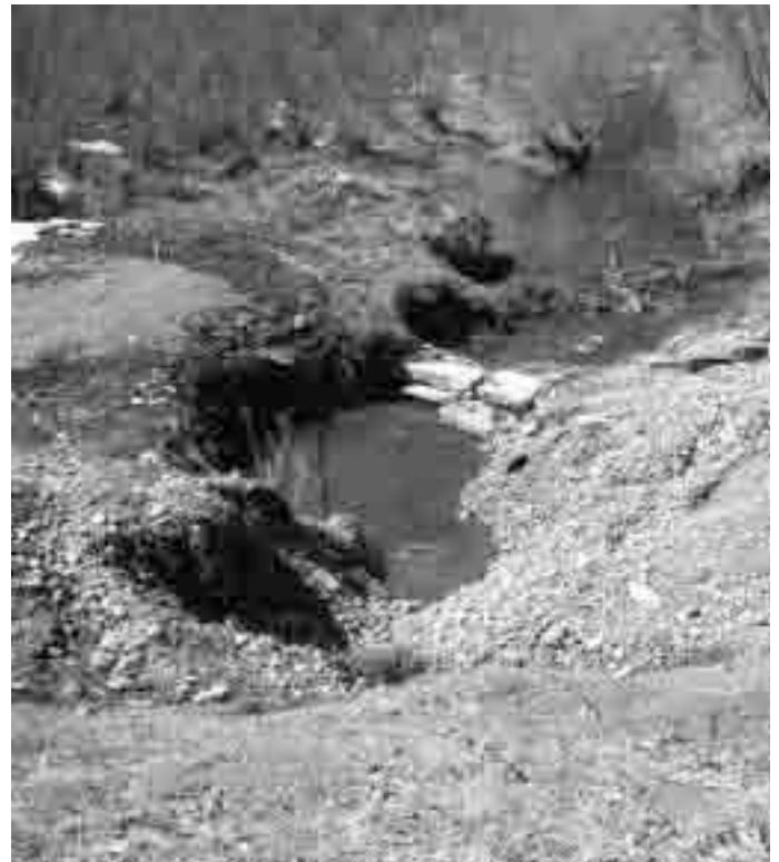
View of the Willow Patch from Mill Street showing excavations recently made by the Village of Cazenovia in order to solve drainage problems with the pipe under Mill Street. This area is the focus of the phase two of improvements and restoration of the Willow Patch.
