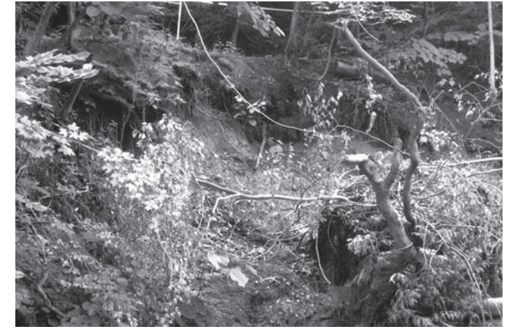
In August, heavy rains and impaired drainage led to a streambank collapse along the Gorge Trail. Repairs required permits, cooperation from adjoining landowners, and $10,000 of CPF reserve funds.
